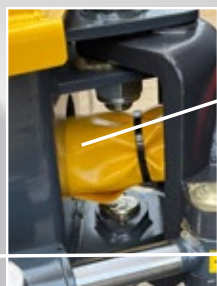
Protected hose lines
